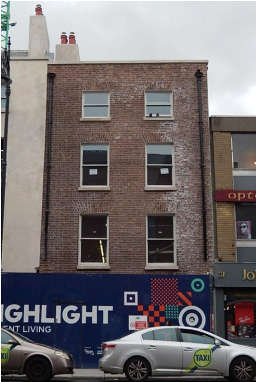
View of newly repointed facade with reinstated wiggled joint and new sash windows
